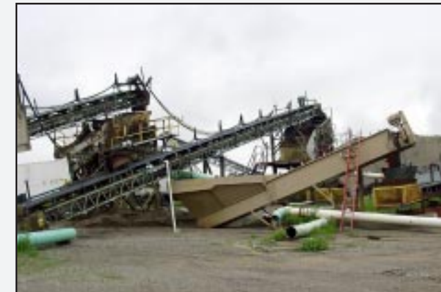
Overview w/ Kolberg E5044 Sand Screw, A-C Screen in Background
